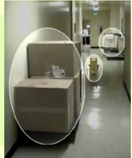
Obstructed exit route
